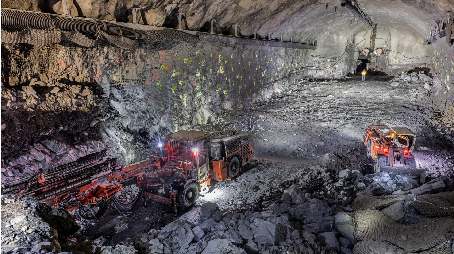
Drilling holes for blast charges for bench C (left) and removing muck (right) in North Detector Cavern (4850-33)
